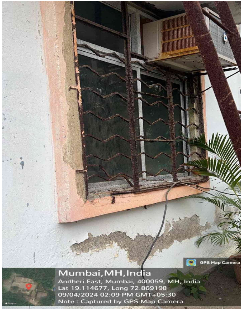
Corroded window grill of the adjacent industry
